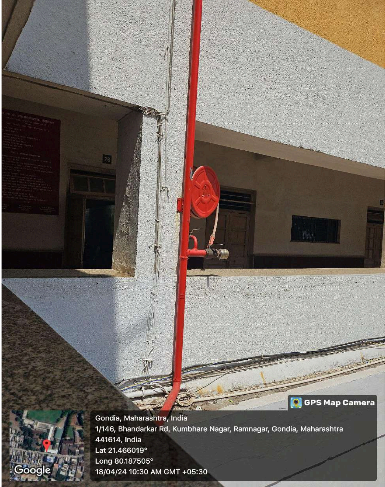
Fire Safety System
